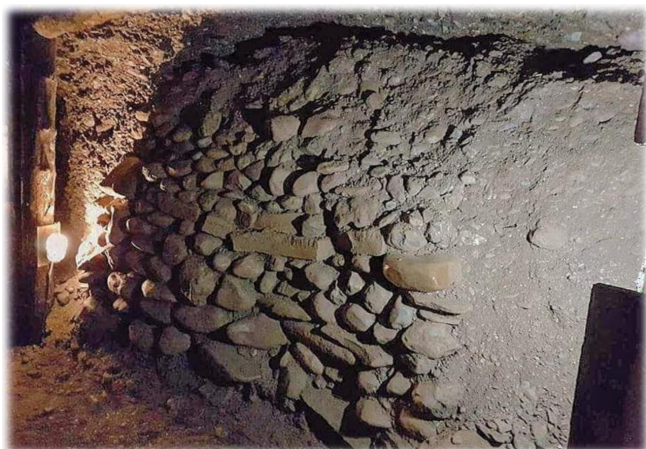
Figure 6. Dry-stone wall constructed within a tunnel passage, composed of river pebbles and used to block or stabilize a sealed section of the underground network.
